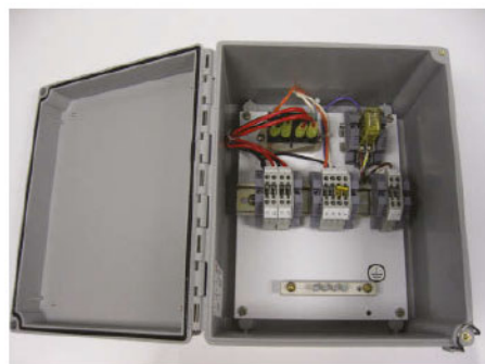
Dump Pump Contractor Panel
