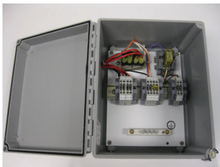
Dump Pump Contractor Panel
