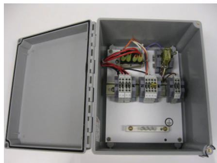
Dump Pump Contractor Panel
