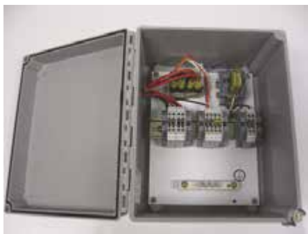
Dump Pump Contractor Panel
