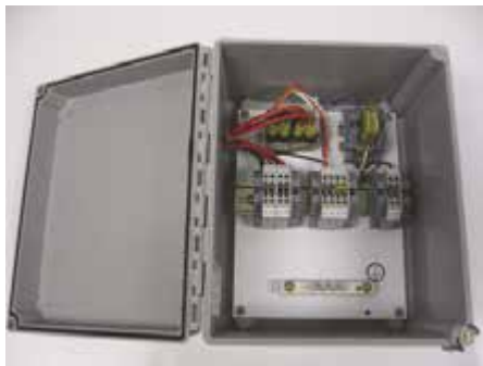
Dump Pump Contractor Panel
